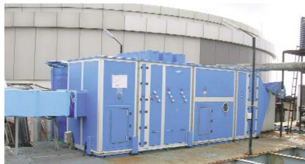
PURAFIL® DBS INSTALLED ON THE ROOFTOP OF THE MINDSPACE
