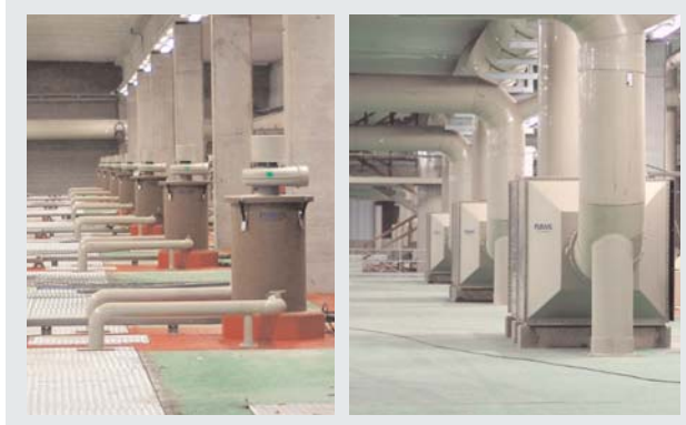
SEVERAL PURAFIL® ESD DRUM-SCRUBBER INSIDE THE BESOS WWTP WORK TOGETHER TO REMOVE THE ODORS FROM THE CITIES' WASTEWATER.
